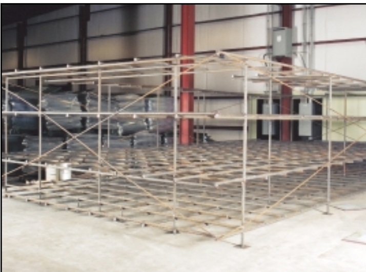
The maintenance personnel at Pax also construct an elaborate re-bar system that will be placed into the pit. The stainless steel tank is placed inside the rebar which will then support the concrete poured into the pit.
