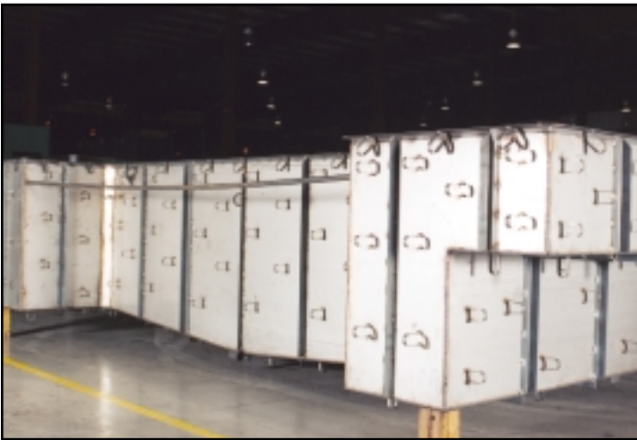
The maintenance personnel at Pax fabricate a stainless steel holding tank for the lubricant. Each tank is custom built to fit the Minster press being installed.
