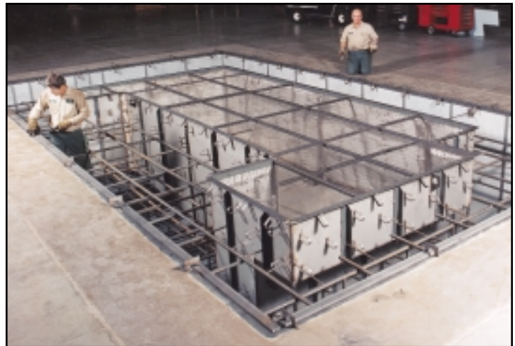
Pax maintenance personnel make final preparations to the press foundation before the concrete is poured.
