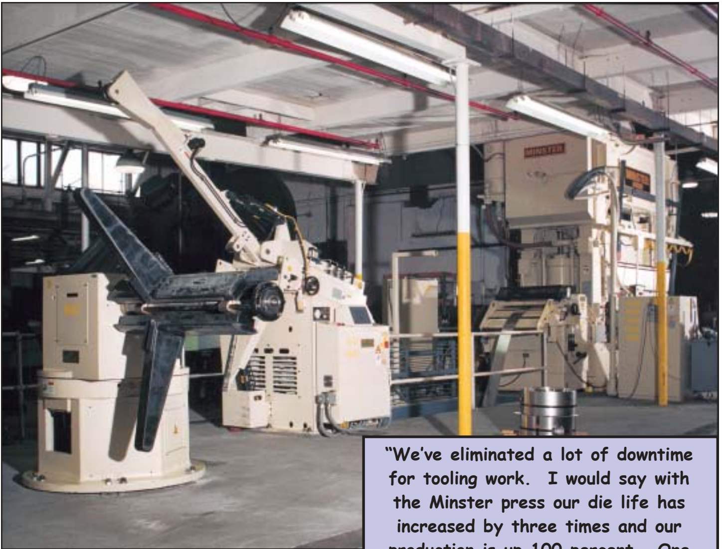
A complete Minster coil line, including a double reel, straightener and feed, are integrated through Minster's Production Management Control (PMC) to optimize productivity at Larson Tool and Stamping.
